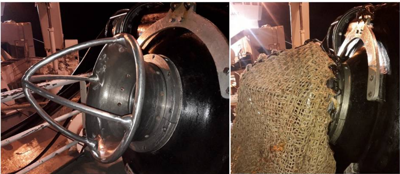
Figure 7.1 - Left: the pump-head funnel; and Right: pump with pump skirt connected [Source: J. Saltskår].
